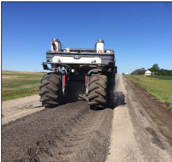
In-place recycling of asphalt pavement and aggregate greatly reduces costs compared to typical reconstruction.
