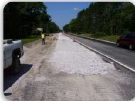
Using performance contracting, the Michigan Department of Transportation rehabilitated an 8.9-km (5.56-mi) stretch of M-115 in Clare County. (Photo Credit: © MDOT).
