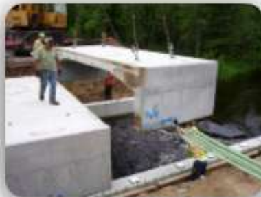
The mid-section of the precast superstructure for a bridge on M-115 is placed as part of the Michigan Department of Transportation's performance contracting project. (Photo Credit: © MDOT).
