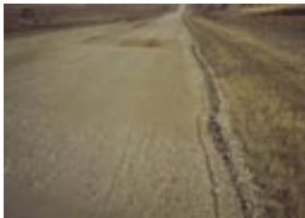
The shoulder problem that develops over time.
