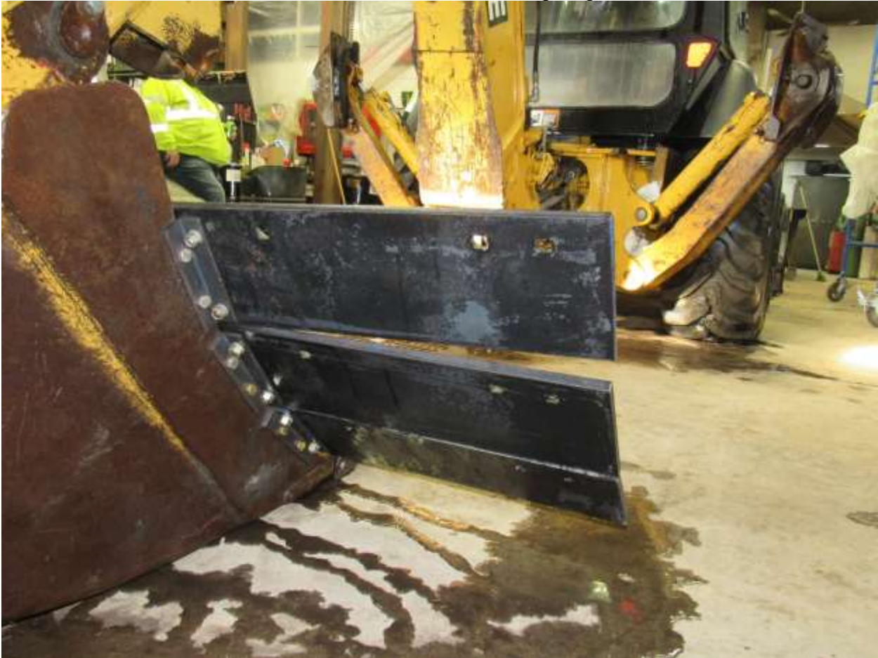
Backside of snow bank buster attached to bucket using angle iron and bolts.
