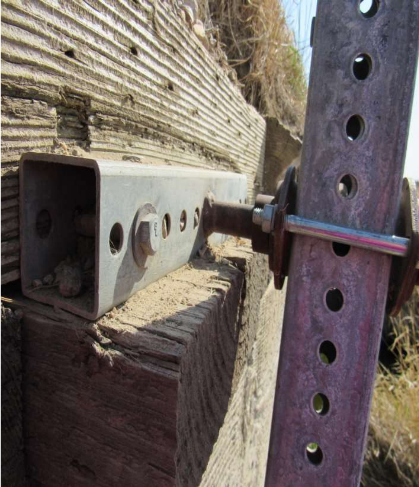
Bridge mount bolted to bridge.
