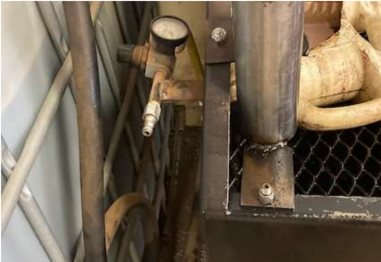
Air compressor connection for air pump.
