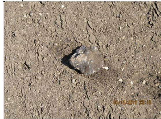
Very hard to avoid a few chunks if pavement is badly deteriorated
