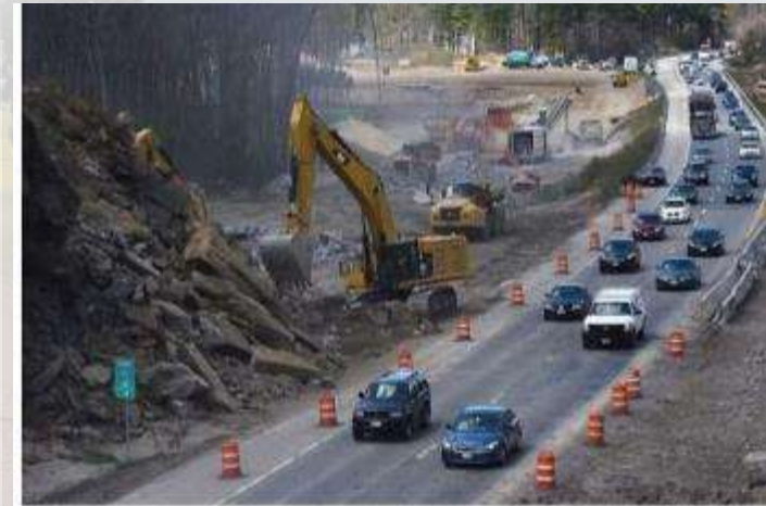
Traffic moves south through a blasting zone, part of the Interstate 93 widening project in Derry. (DAVID LANE/UNION LEADER)
